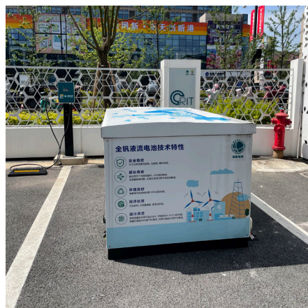
The solar fence and energy storage batteries in Hangzhou, China.
